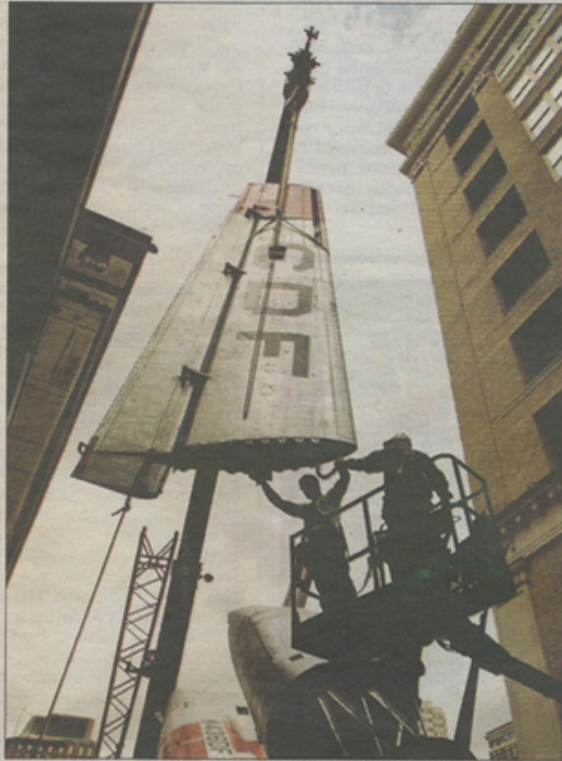
Artist Jordan Griska (left) and ironworker Eddie Bell position wing of a Gruman Tracker II aircraft, which will be an exhibit at Lenfest Plaza, a new civic space at Broad and Cherry streets.
